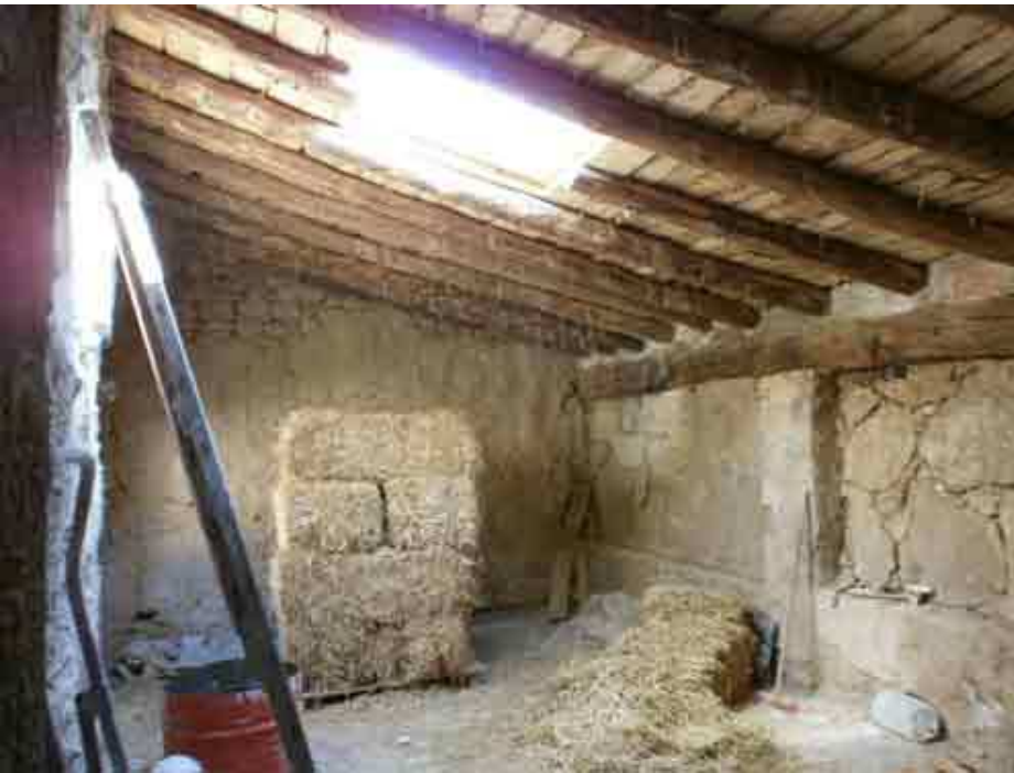
The part from which the roof that has been rebuild, with a earth/straw insulation.
